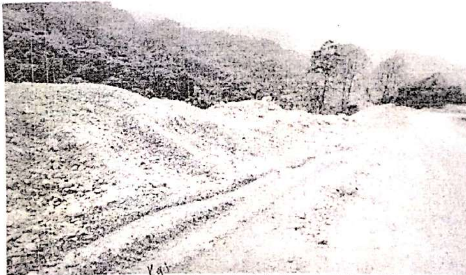
Picture:4 The muck being along the road side in flagrant violation of Muck Disposal Plan issued to Shivam Trans Construction Private Limited. These muck roll down the hilly slope and also the dust emitted from these muck make the life of commuters a hell.
