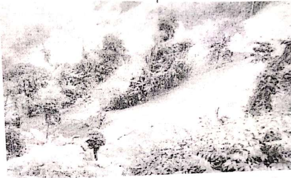
Picture-1. Indiscriminate dumping of muck/debris in the project site by Shivam Trans Construction Private Limited. The muck/debris are seen rolling down the hill slopes in total violation of the guidelines of the Forest Clearance and making a mockery of the Designated Dumping site guidelines.
